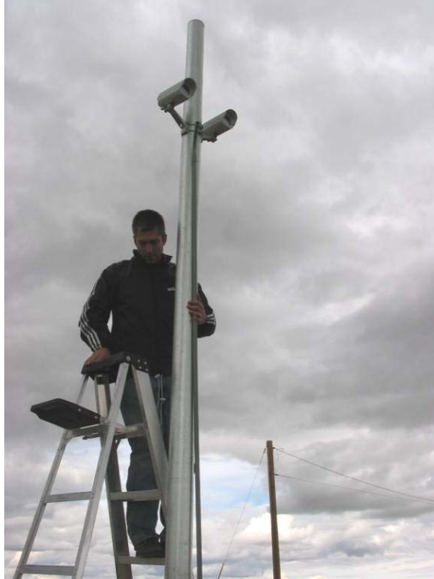
Figure 3.8: System 1 (Xtralis 7) and System 2 (Xtralis 5-6) mounted on the same pole (Photo: Matt Blank, WTI/MSU).
